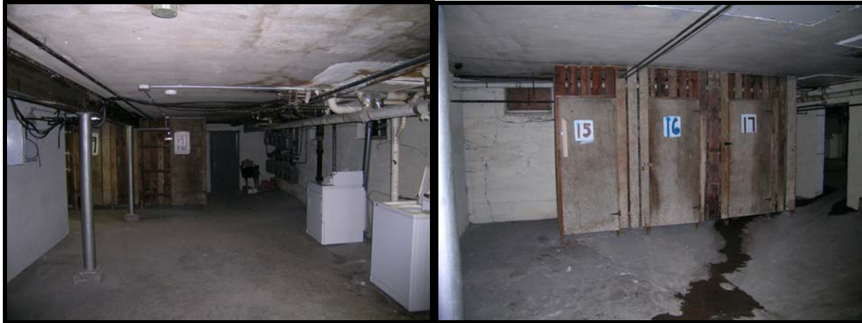
PHOTO 5. BASEMENT AT 1206 DEWEY
