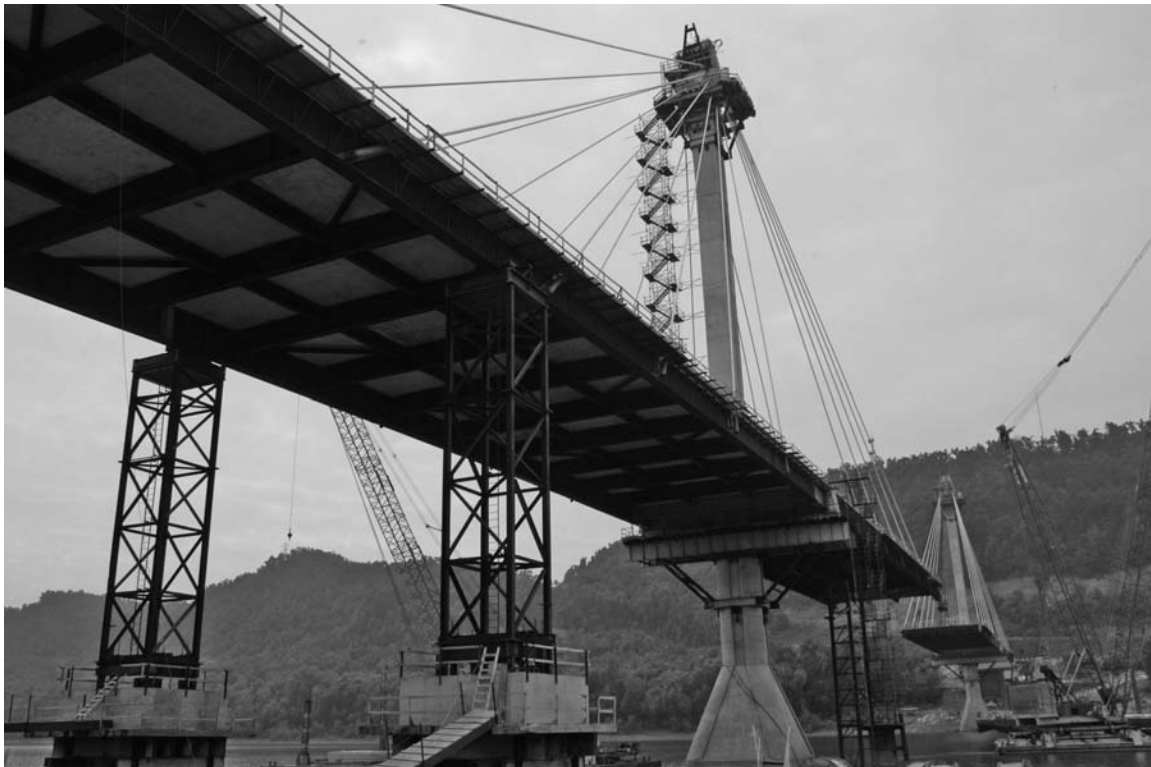
Figure 3: The partially completed US Grant Bridge. As viewed from the North, August 2005.
