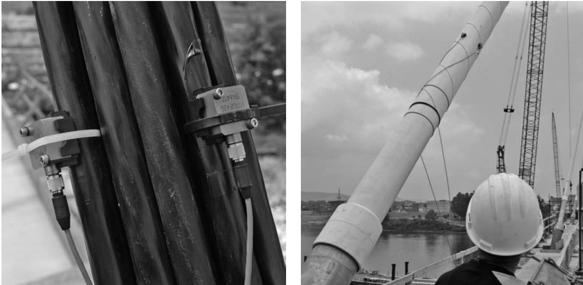
Figure 2: Accelerometers mounted on a US Grant Cable Stay (left) and Stay Sheath (right)
